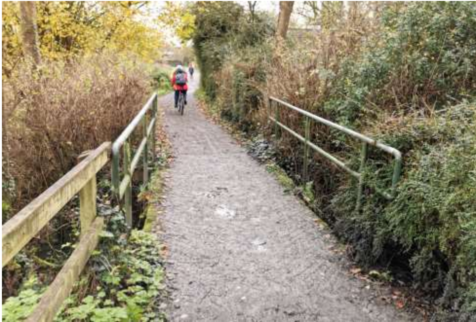
Figure 6-27: Existing bridge (Bridge 4) over the decommissioned and dry Plassey Mill race overspill
