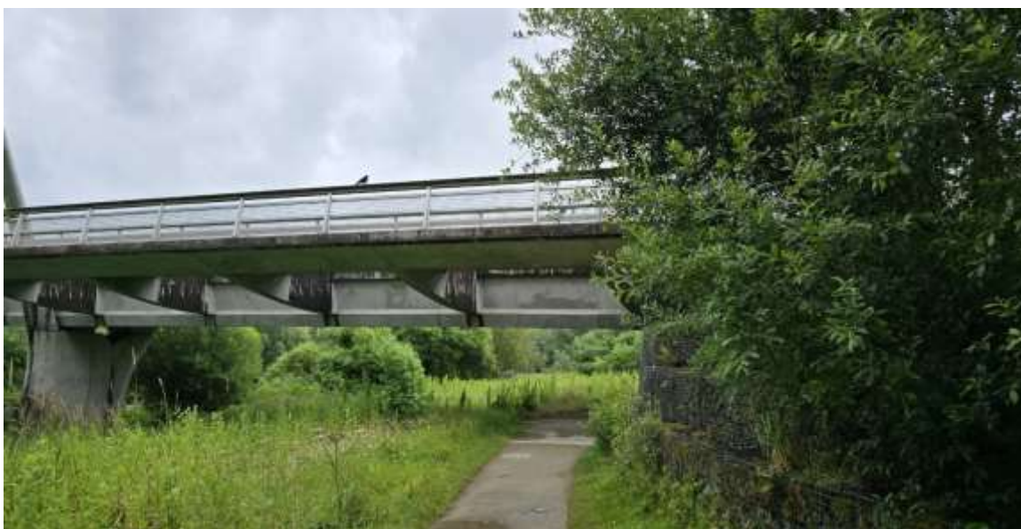
Figure 6-35: Existing road bridge between the UL campus in Co. Limerick and Co. Clare
