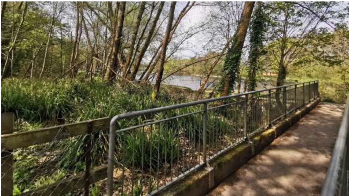
Figure 6-49: Existing concrete bridge at mouth of Plassey mill race with Plassey Beach in the background
