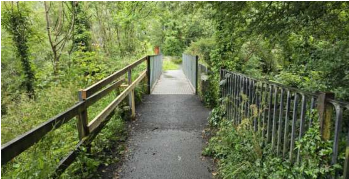
Figure 6-20: Existing temporary bridge across the Plassey mill race where it rejoins the River Shannon
